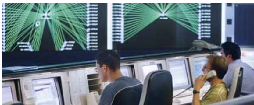
A central control room is the hub of the fire prevention concept
